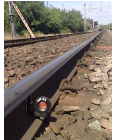
Pictured above: One of the 300 mini prisms fixed to the rails to monitor the track.
